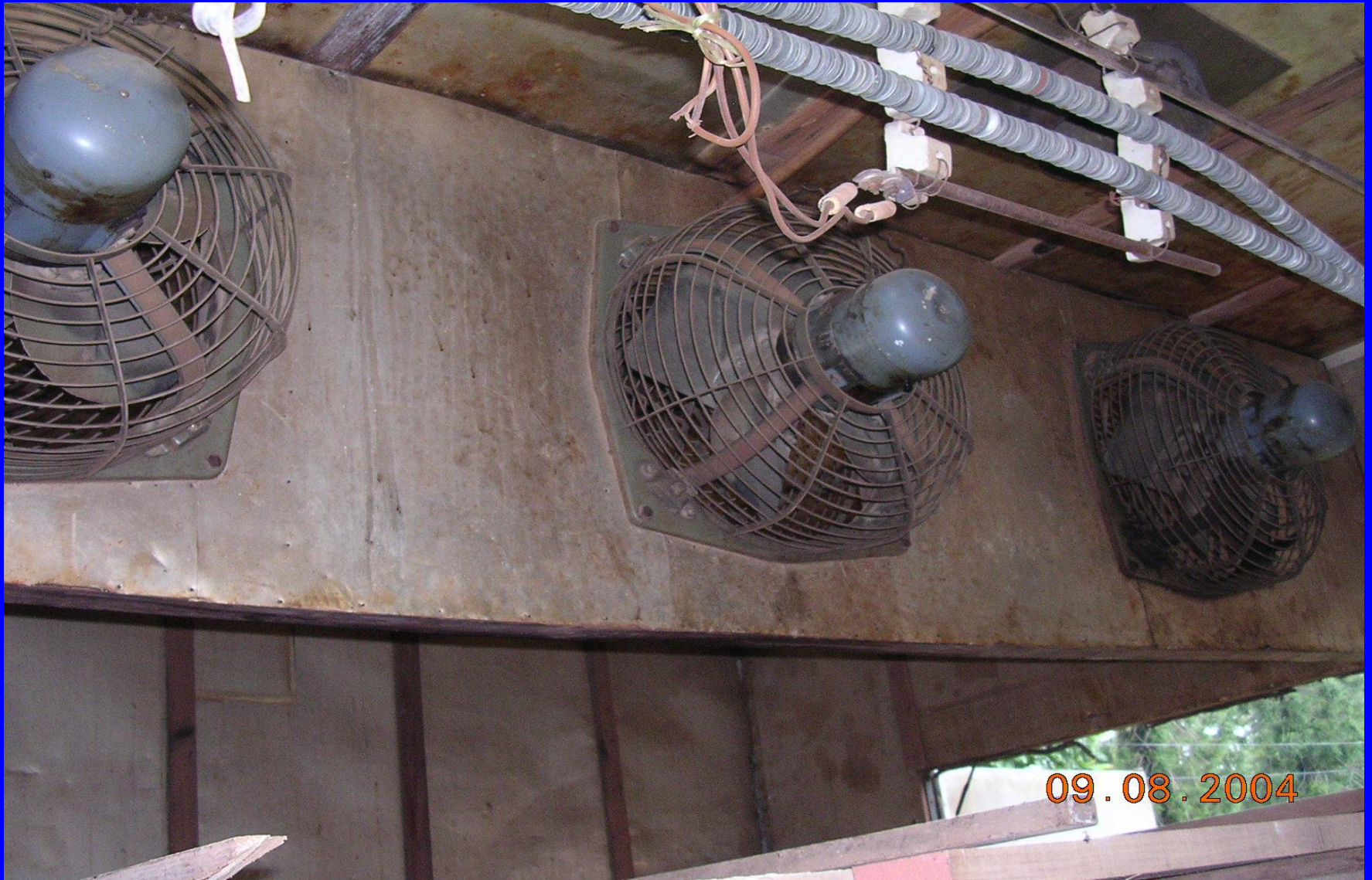
Fans and electrical heaters
