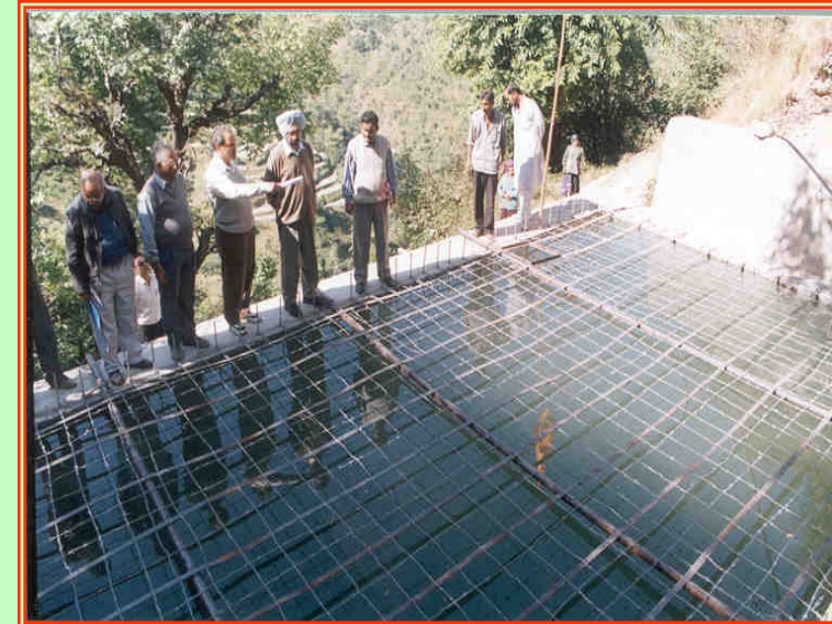
Delegates of World Bank Team visiting RCC irrigation tank at Sainji
