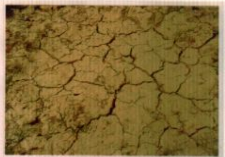
Cracks during summer period
