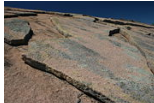
Effect of Weathering on Granite
