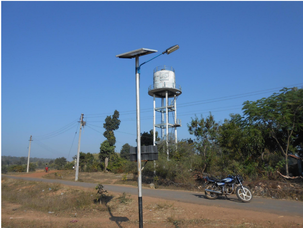
Solar Street Light - 1451
